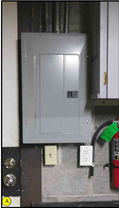
NEW CIRCUIT BREAKER PANEL Inside the Maintenance Building
