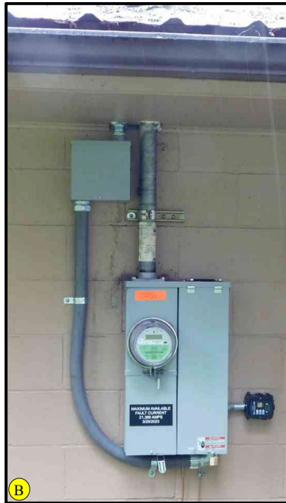
NEW ELECTRIC METER/BOX On South Side of Maintenance Building
